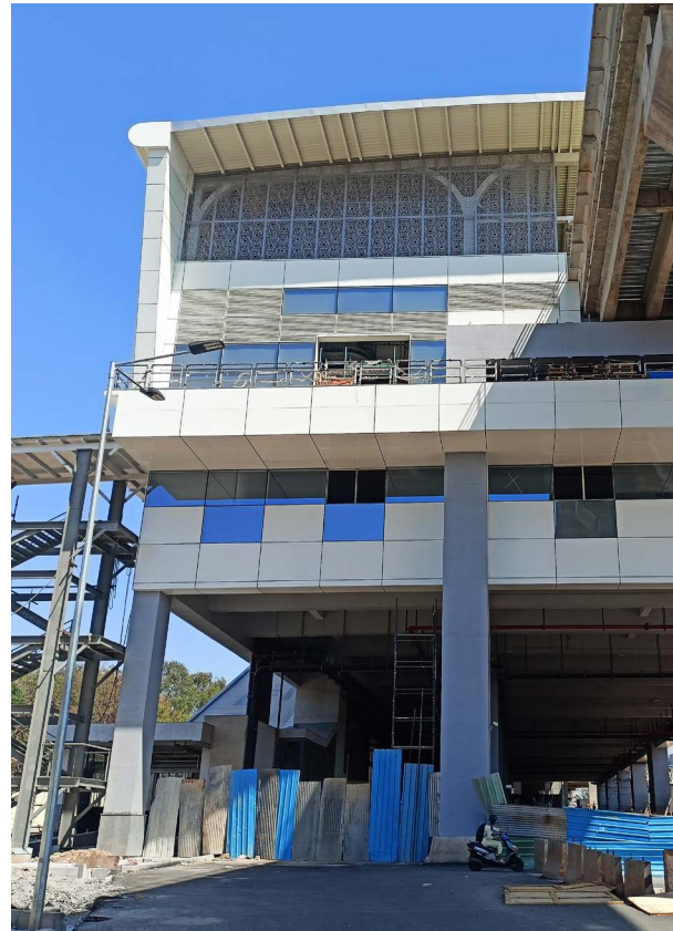
Infosys Foundation partnered with Namma Metro to construct a metro station in Electronic City, which will be one of the city's LEED-certified stations under the Indian Green Building Council (IGBC) Green Existing Mass Rapid Transport System.
