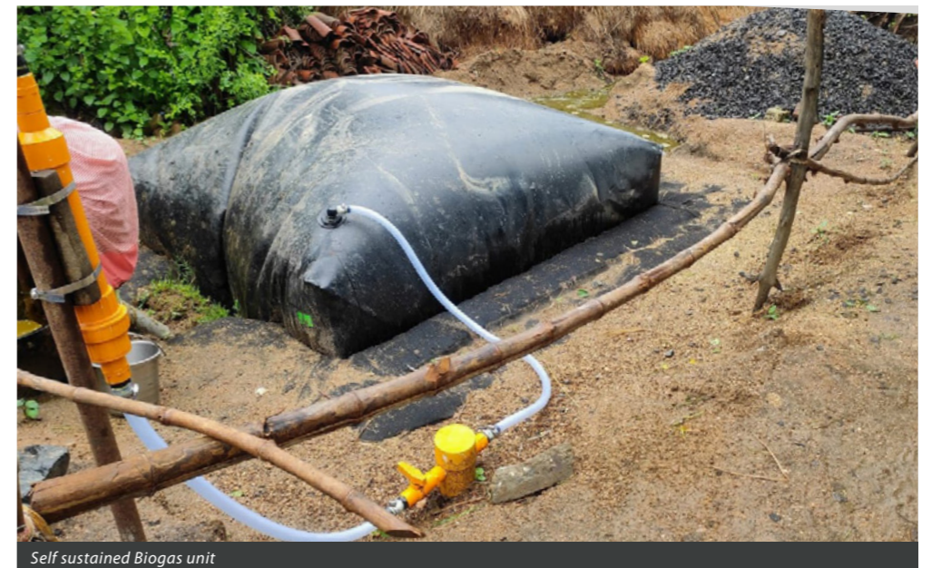
Self sustained Biogas unit
