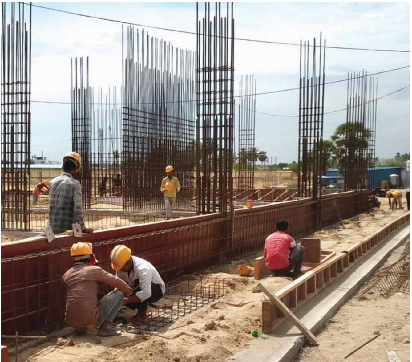
The Infosys Foundation Girls Hostel is being constructed at IIIT Trichy's new campus at Sethurappatti.
