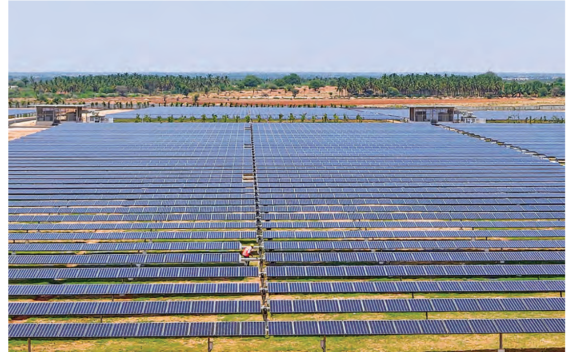
40 MW solar plant in Sira, Karnataka
