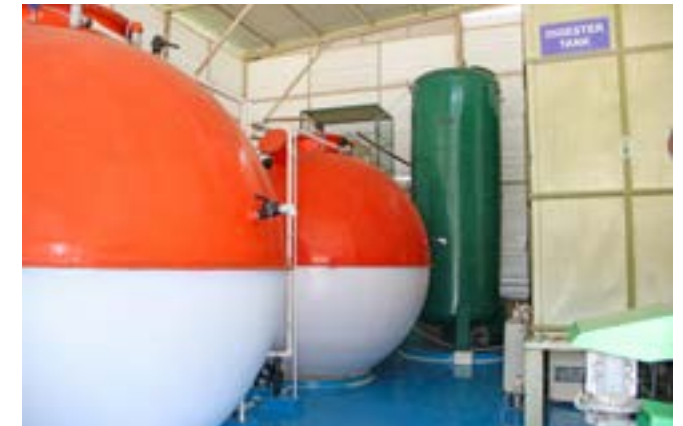
Biogas plant at an Infosys campus
