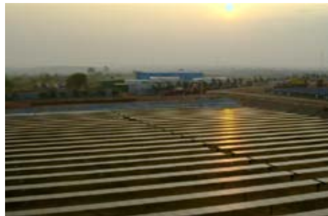
Solar plant in Sira, Karnataka
