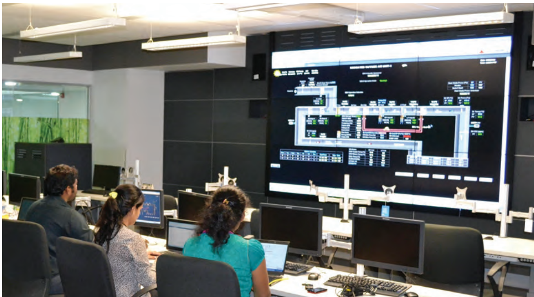
The Infosys Command Center in Bangalore manages about 45 million sq. ft. of area across our campuses
