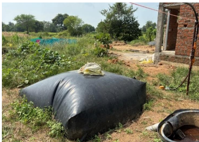
Figure 133: Digester of the biogas unit
