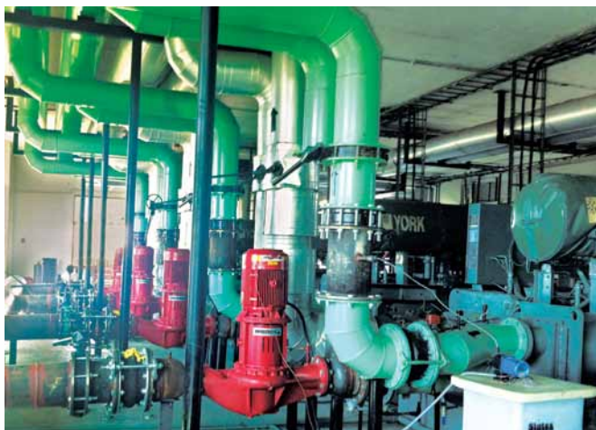
Figure 5: End-suction pumps – before retrofit
