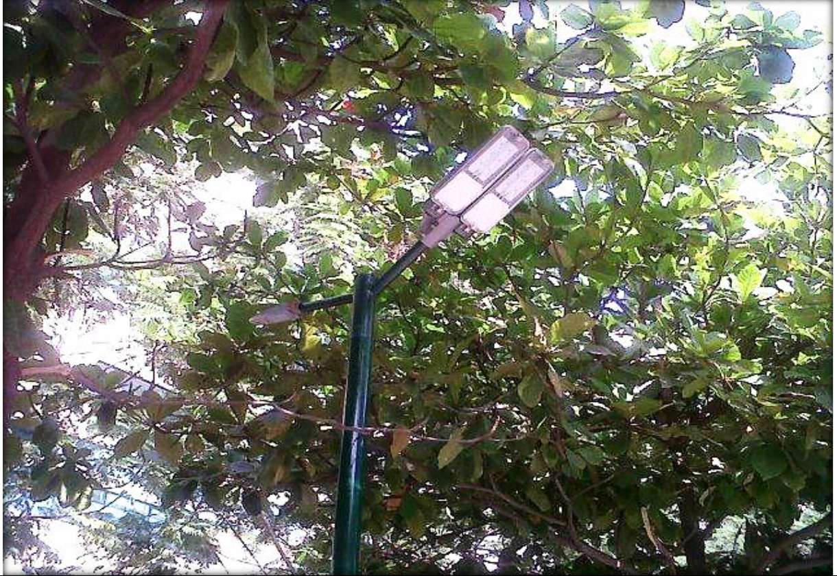
Energy conservation measures solar panels
