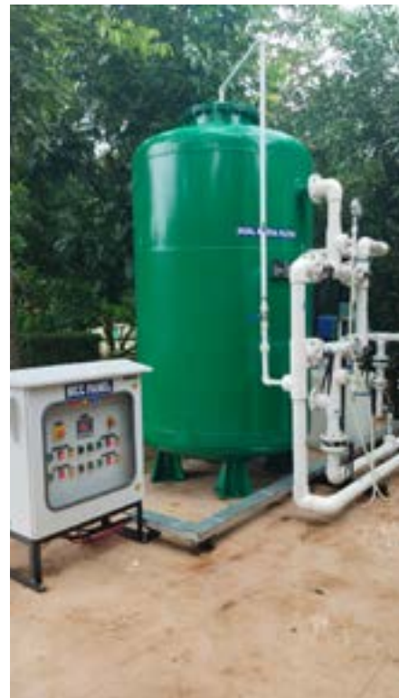
Filtration system to treat the rooftop rainwater before reuse.
