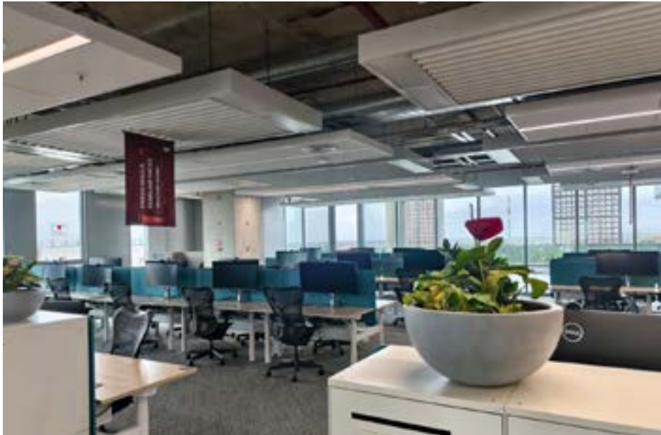
Infosys' Radiflux radiant cooling solution integrates digital monitoring with existing infrastructure.
