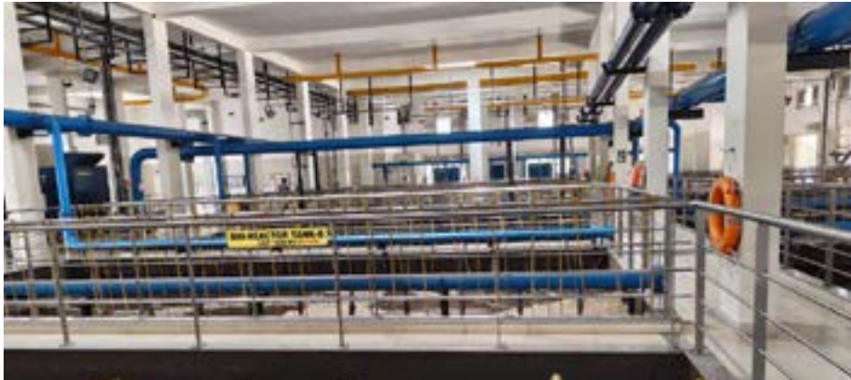
Infosys uses advanced membrane bioreactor technology in Sewage Treatment Plants to treat wastewater.
