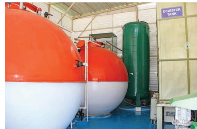
Biogas plant at an Infosys campus
